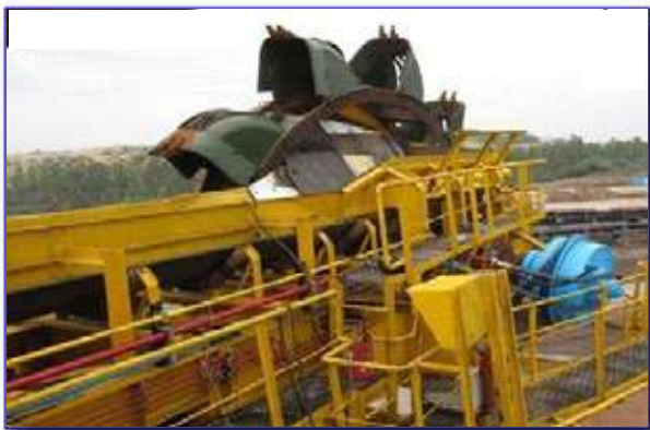
4000 TPH Bucket Wheel Reclaimer Drive
