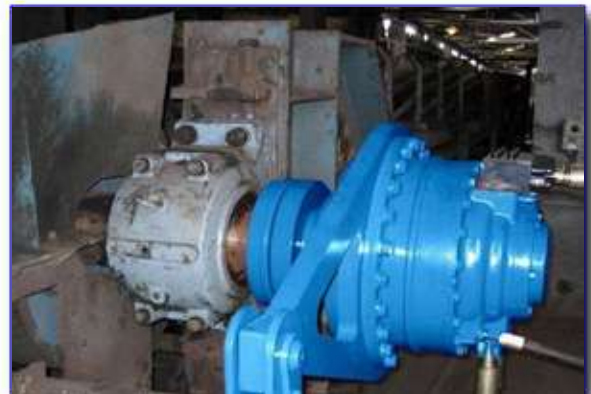
2000 TPH Conveyor Drive Conversion
